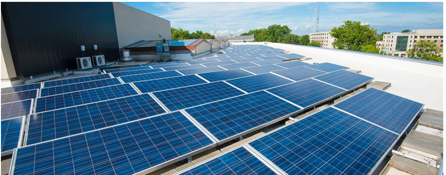
Rooftop solar panels at AU.
